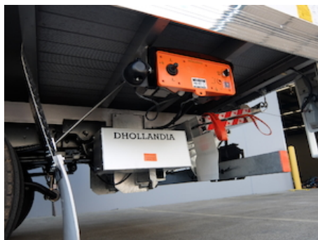
Electrical controls without sensitive electronic components
