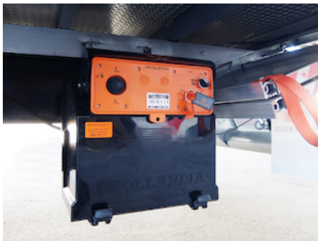
Electrical controls without sensitive electronic components
